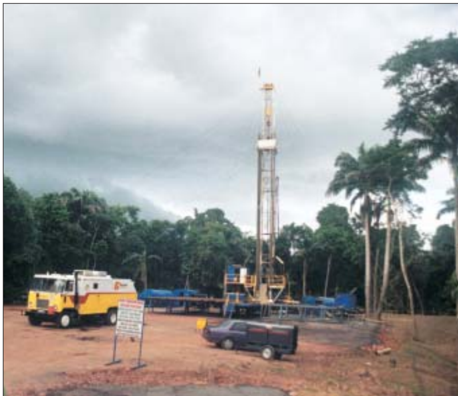
New Horizon Exploration Trinidad & Tobago Ltd.'s "Rosie" drilling rig prepares to spud Well No. 19 on the first Six-Pac pattern on the company's Parrylands Block E in Trinidad.
